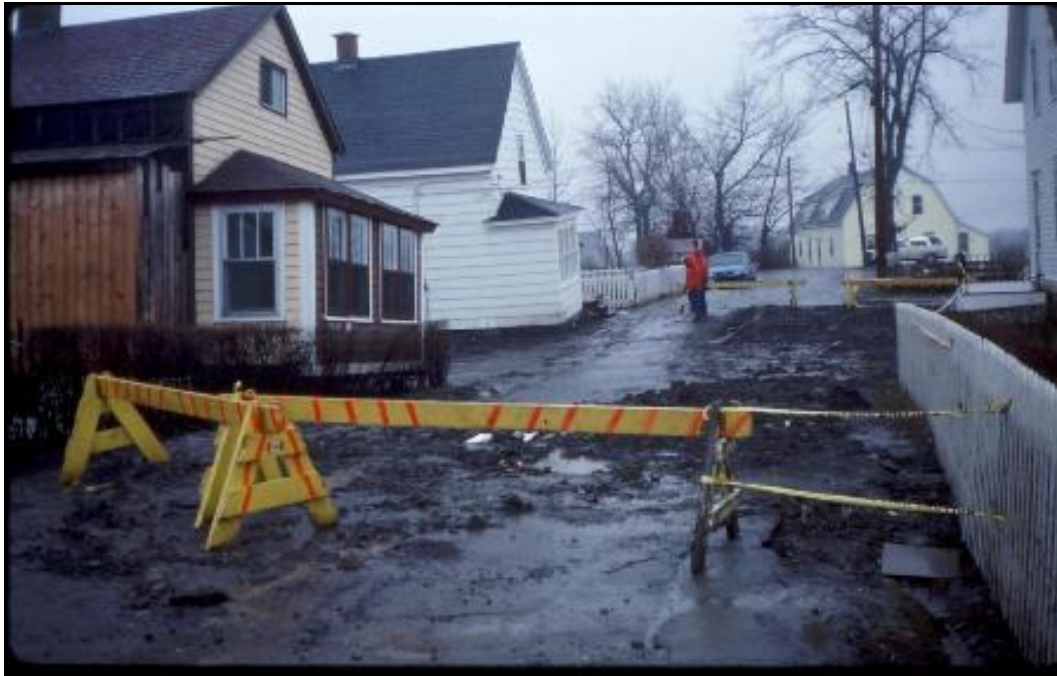
Photo 7: Settling houses over underground coal workings, Nova Scotia.
